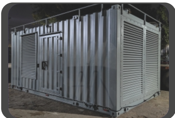
20' EMI / EMC CONTAINER (500KVA)
