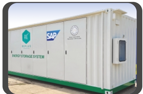
30' HIGH CUBIC BESS CONTAINER
