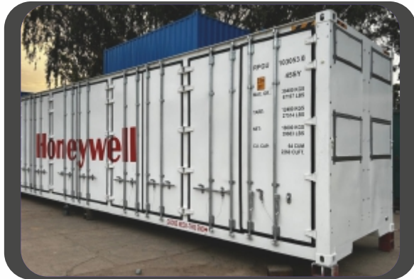
40' HIGH CUBIC BESS CONTAINER
